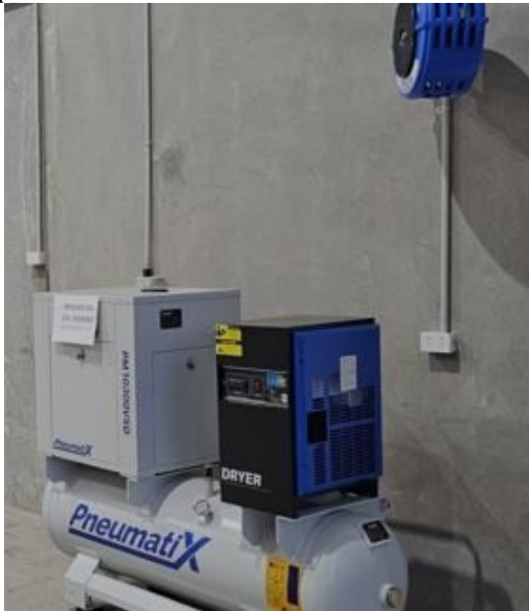
Photo 1 - Typical overview of power outlets and compressor positioning.
